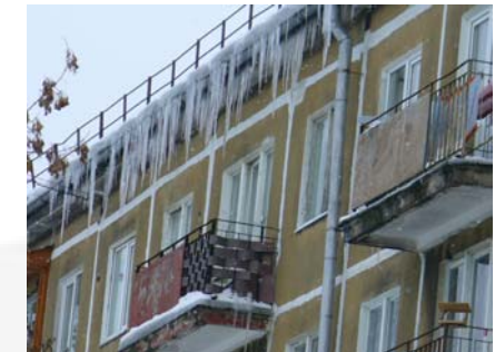
Pic.13, intensive heat losses (a multi-apartment building in Jugla). [2]
