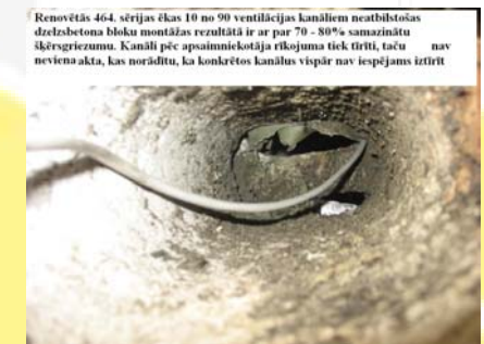
Pic.15, ventilation shaft with a construction defect (multi-apartment building of series No.464). [7]
