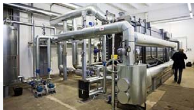
Pic.26, Absorption heat pump in CHP plant "Imanta" in Riga
